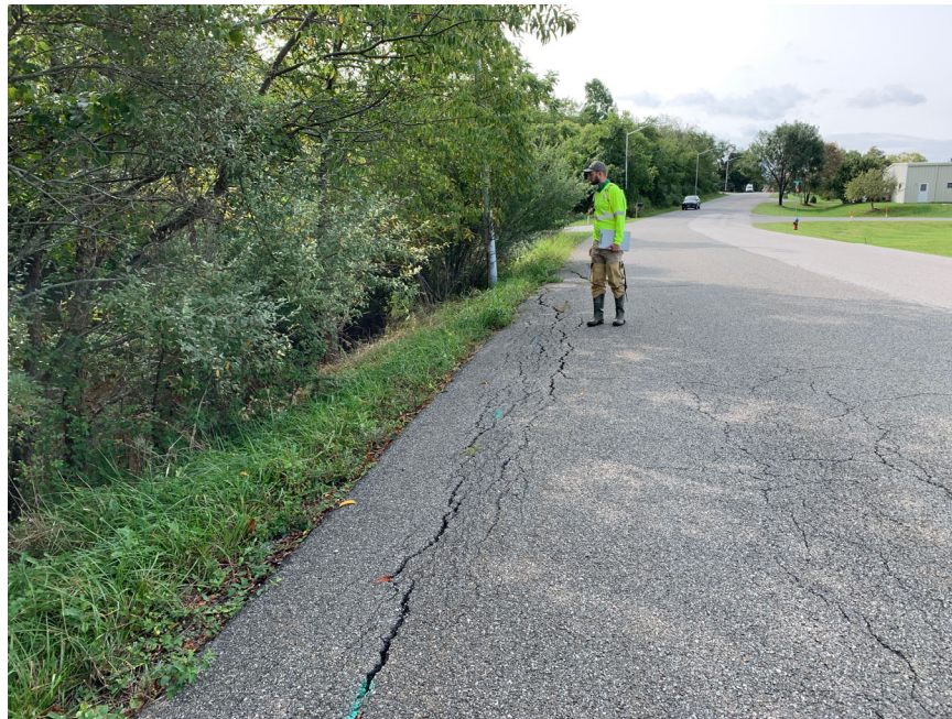
Figure 3. Cracking in the asphalt making up Industrial Drive NE, the 60-inch outfall originates below the left shoulder and flows into the foreground, green striping marks the 8-inch sanitary.
