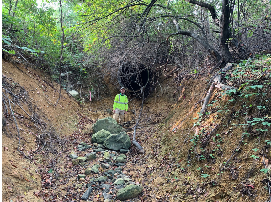
Figure 2. 60-inch culvert outfall, severe downcutting can be seen (approximately 4 feet), Industrial Drive NE is above the right bank.
