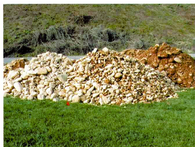
As part of the stream restoration, a specially designed stream bed mix was installed to improve stream bed stability.
