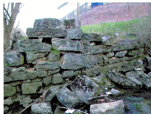
Remnants of a stone wall believed to be from Wade's Mill, mid-19th century, can still be seen along the stream bank.
