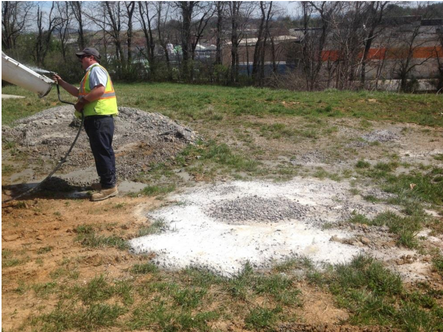
Photo 1. March 23, 2016. Illicit Washout in Progress. Driver was directed to the existing concrete washout constructed at 405 Roudabush Drive. Driver was unaware of the washout location
