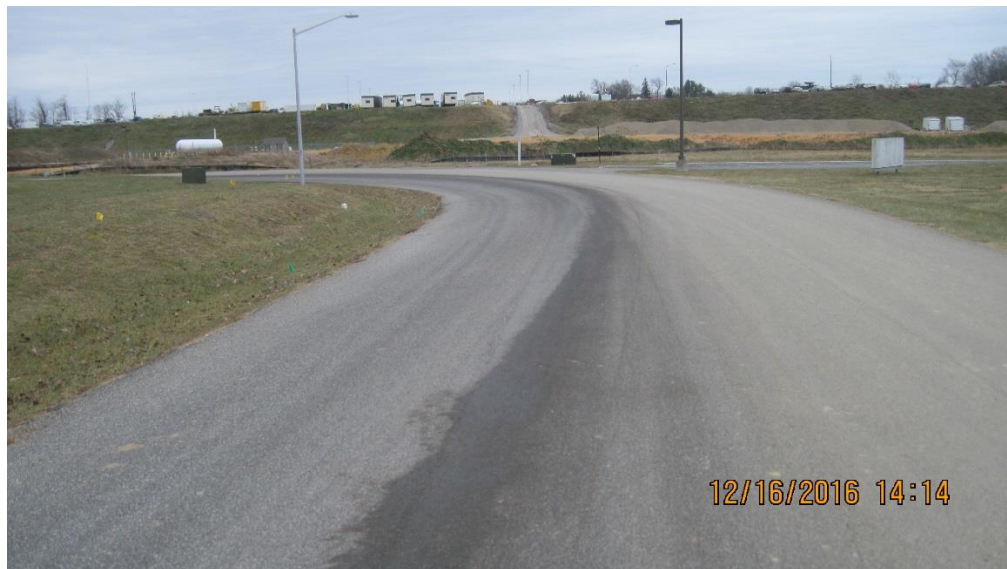
Photo 1. December 16, 2016. Hydraulic line spill after sorbent application.
