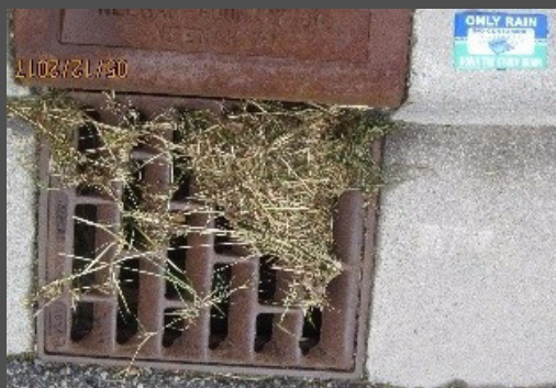
Grass clippings stuck in a storm drain.
