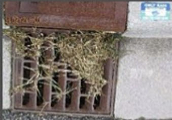
Grass clippings stuck in a storm drain.
