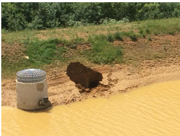
Photo 1. 5/26/17. Sediment Basin outlet pipe piping failure.
