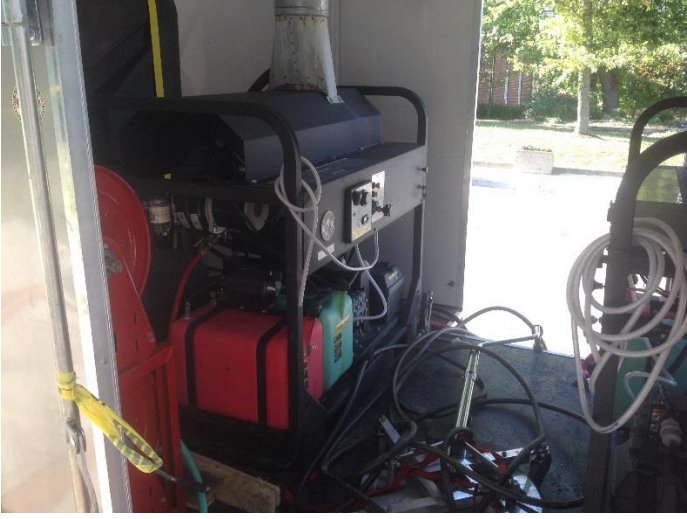
Photo 4. October 24, 2016. Interior of filtering equipment trailer.
