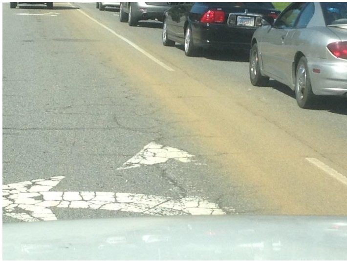
Photo 1. October 19, 2016. Sediment tracking on North franklin Street south of the Depot Street Intersection.
