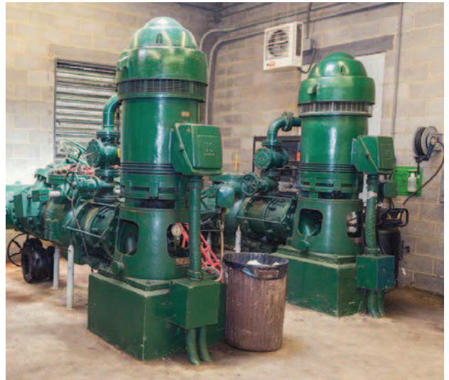
Pictured are two of the plant's water pumps. The pumps draw water from the New River to the treatment plant.
