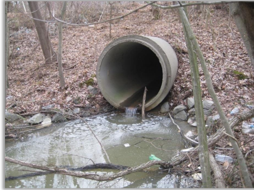
Figure 2. This manual aims to prevent pollutants from entering stormwater conveyances and ultimately receiving waters.
